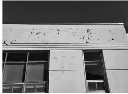
The capital reserve fund, if approved, will address peeling exterior paint that exposes masonry to moisture, increasing the risk of water infiltration and long-term damage to the building structure.
