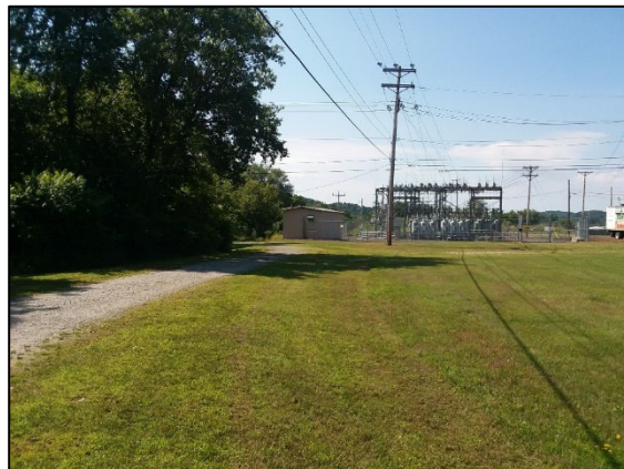
Figure 12: Electrical substation and overhead power lines
